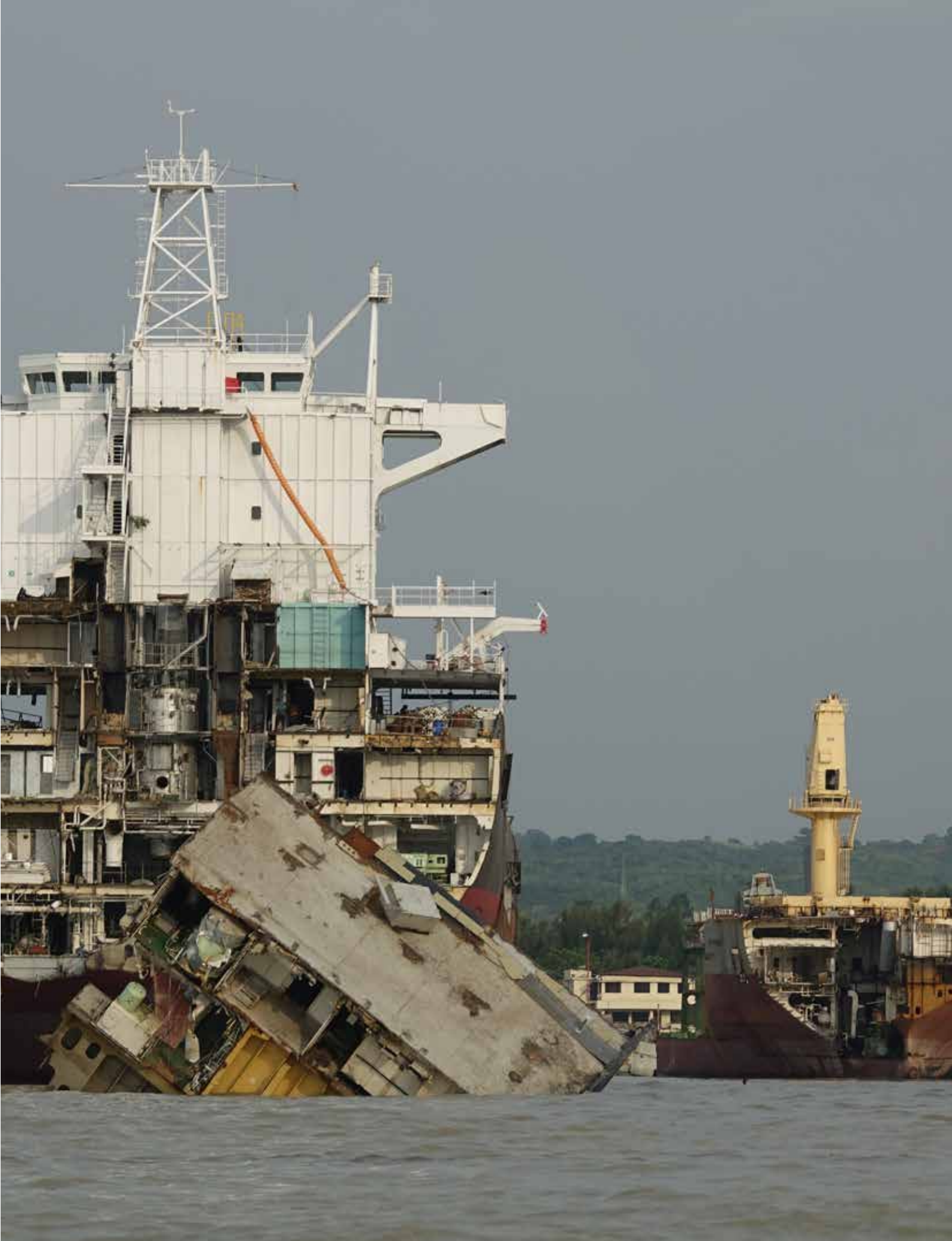
When a ship is dismantled the so-called 'gravity'-method is used where large blocks are cut off the hull and fall down onto the sea bed. Afterwards the blocks are broken up further until they are small enough to pull ashore..
